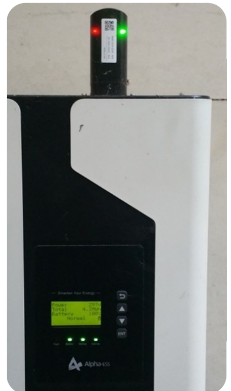
Solar energy system by Lisa, Greensborough
