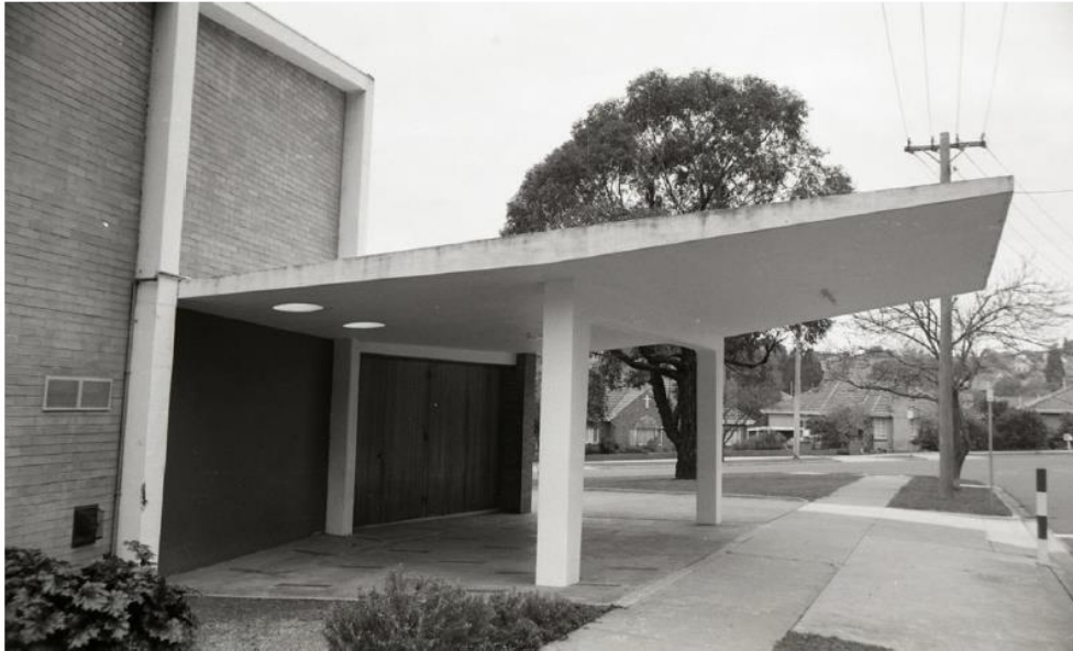
Close-up of cantilevered porch, mid-1980s – soon after partly enclosed with glazing, mid-1980s Note original floor of white Carborundum (silicon carbide stone) panels and 'English' grey-blue quarry tiles The mature tree central to the triangular front garden (background) has since been replaced (Source: courtesy of Graeme Butler)
