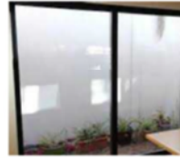
014 - aluminium framed windows with clear glass Powder coat finish (black) - colour to be confirmed
