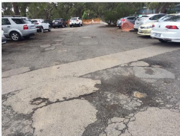
Figure 5: Looking east within the site showing state of car park surface
